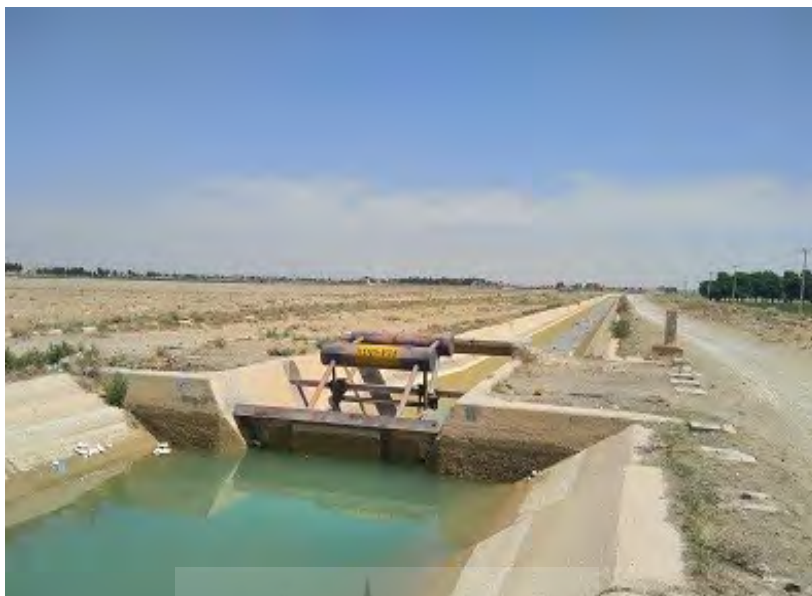
Fig.4. A valve divides the water between South Baraan village and the downstream village. A guard is assigned in this area to take care of the water distribution. Water theft from the village occurs when someone secretly opens the valve and redirects the water to the downstream village. Source: field observations
