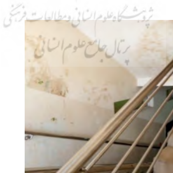
Fig. 13: Traces of Spirogyra and dampness noticed on the wall and underneath the staircase due to poor position or maintenance of the water reservoir
