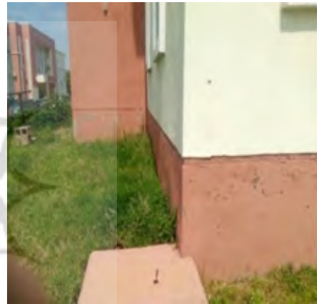
Fig. 12: Painting on the wall of the building pilling off.
