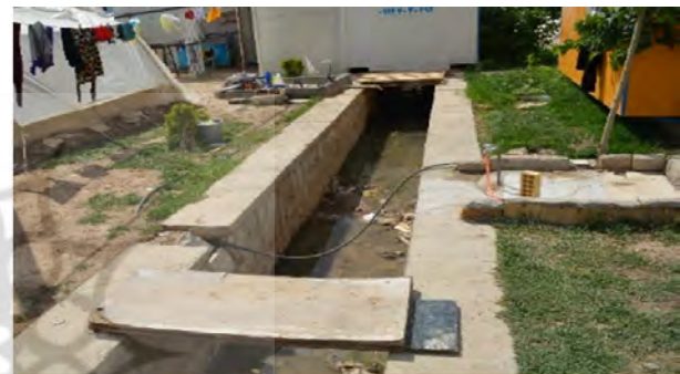
Figure 18. Clogging of water in canals (Source: Authors)
