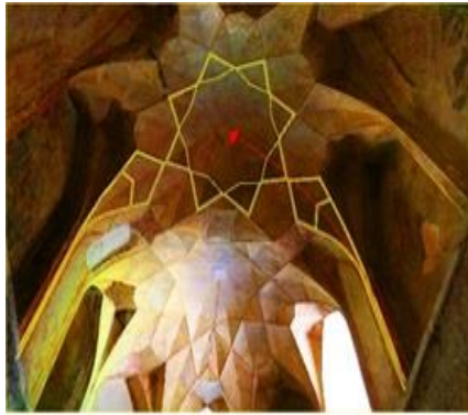
Figure 12. The use of branches in a coordinated geometric structure. Part of the roof covering and decorations of the Qazvin Pergola Mansion. Source: Author.
