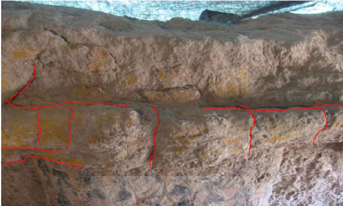
Fig. 9. Parallel cracks in forearm of statue and separation of chest and waist scarf due to wet to dry contraction of clay mud (author, 2006).
