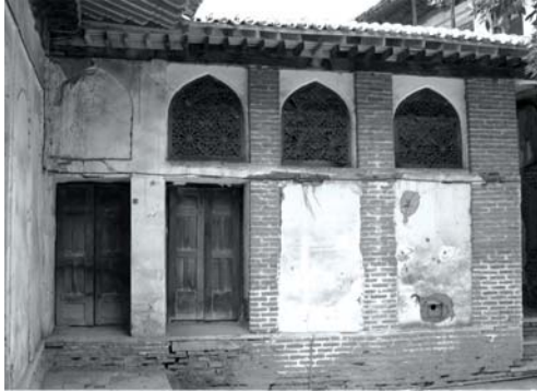
Fig. 11: Blocked openings in the first family courtyard and samples of existing and blocked herringbone windows
