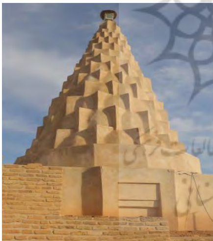
Fig.10. The chipped dome of the building
