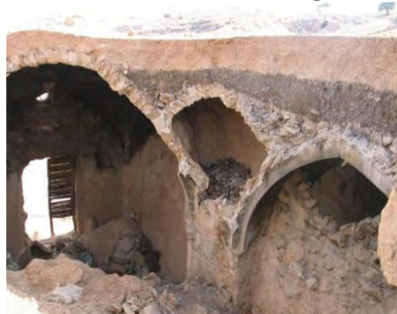
Fig.22. Layers of covering between the arch and the roof in one of the villages of Shushtar city (Chaharmahali, 2016)
