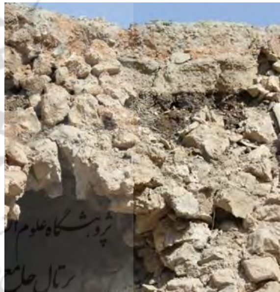
Fig.21. The four layers of roof water isolation and the arches below it are shown in the figure
