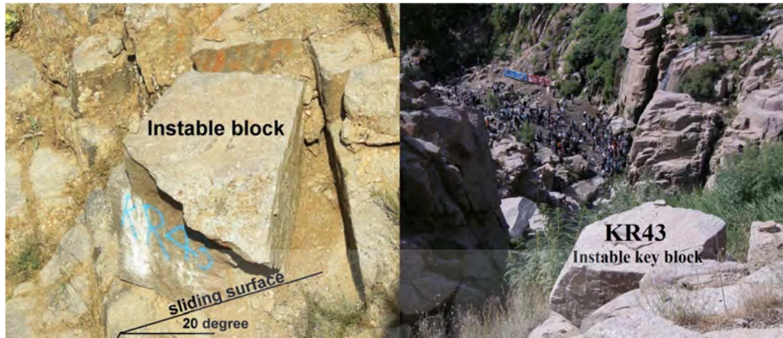
Fig. 6: A view of key block KR43 detaching due to Ice jacking action
