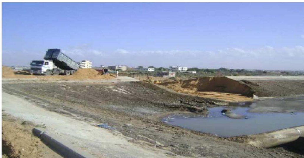
Figure 14 Damage to an anaerobic pond in Gaza Wastewater Treatment Plant caused by the recent Israeli invasion, 2009 (Photograph by Fareed Ashour)
