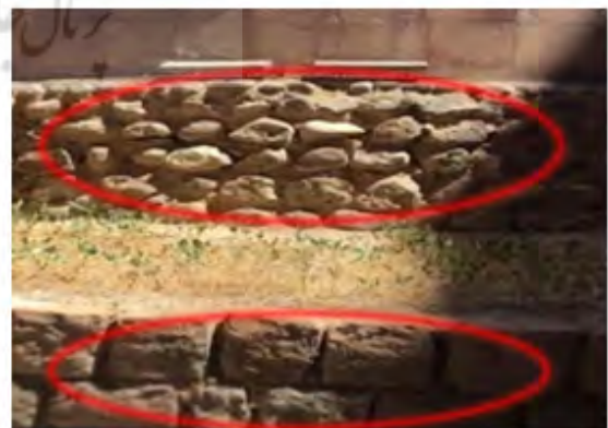
Fig. 12: Evidence of the use of rubble and cut stones in the basement of the building
