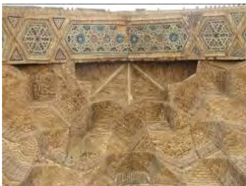
Fig. 9: Moqarnas and geometric ornaments under the outer arch of the southern iwan
