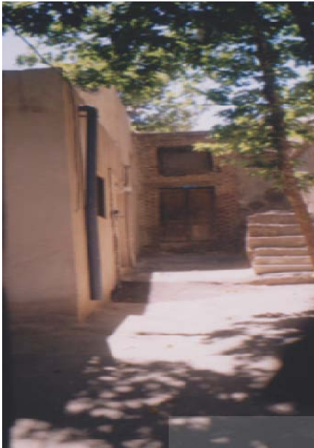
Fig. 5: very eroded dwelling house wooden entrance and stair of its adjacent eroded house in Hasanabad zargande, region 3 of Tehran municipality. (Source Authors)
