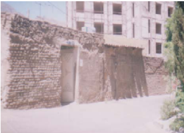
Fig. 3: Ab eroded dwelling house adjacent to a 5-floor building which is in construction process in Gheitariyh district, region 3 of Tehran municipality (the installed cooler in the eroded house indicates that the house is being used). (Source Authors)
