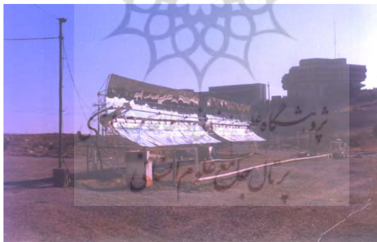
Fig.2-Typical view of the collector installed north-south direction
